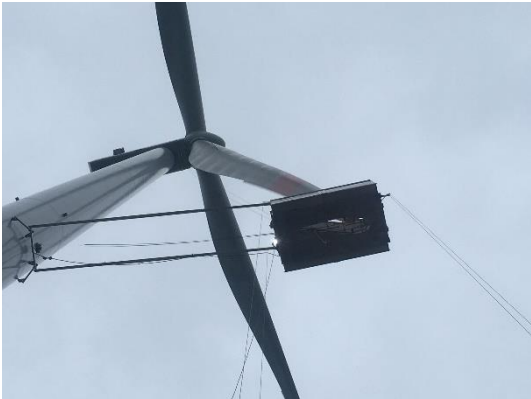
SYSTEM terra in operation on a V150 Vestas turbine © WP Systems GmbH
